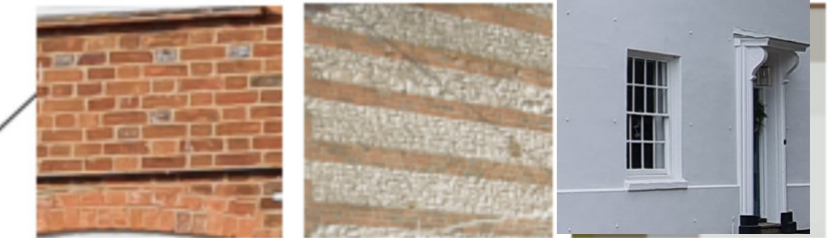
Handmade facing brickwork - Berkshire red / including use of burnt or vitrified headers
