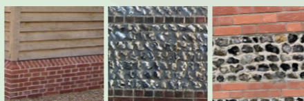
Plinths and Boundary Walls - brick plinths with timber cladding atop. Boundary walls in brick, brick and flint or Brick and local stone
