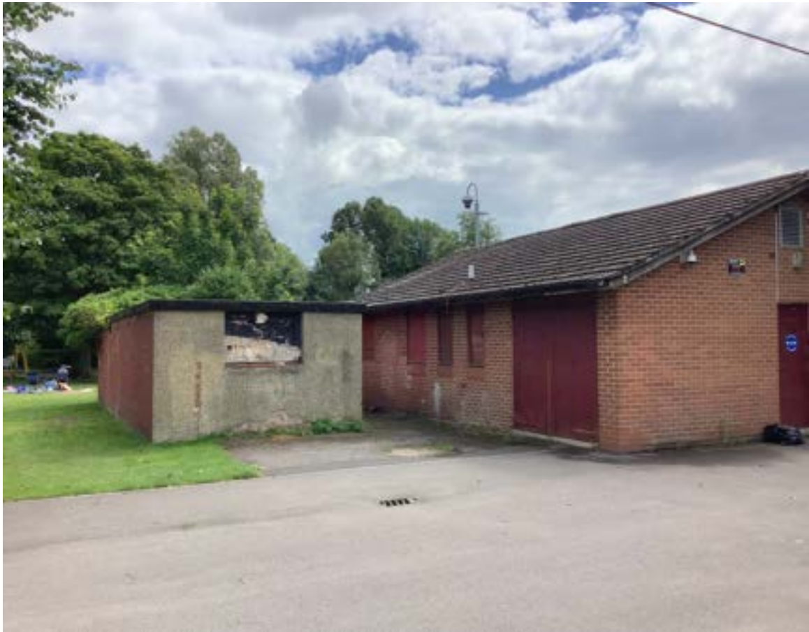
Figure 133: Poor quality structures on the western side of Victoria Park near the play area. The smaller building on the left (due for demolition), was a Second World War air raid shelter that served the nearby nursery.
