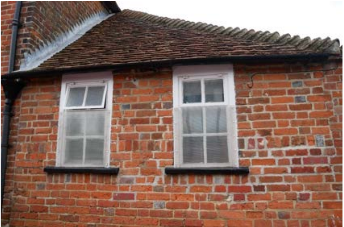
Figure 246: Unattractive and intrusive intervention into historic windows at the rear of St Bartholomew's Hospital Almshouses.
