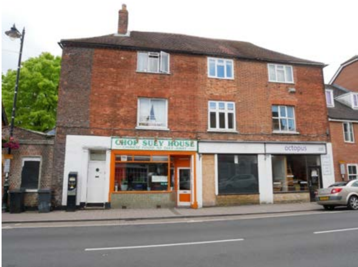
Figure 116: Modern windows and a loss of original features on a historic building on Bartholomew Street.
