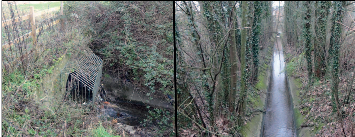
Figure 2.2: Thames Water sewer emerging from culvert (left) and concrete channel on-site (right)
