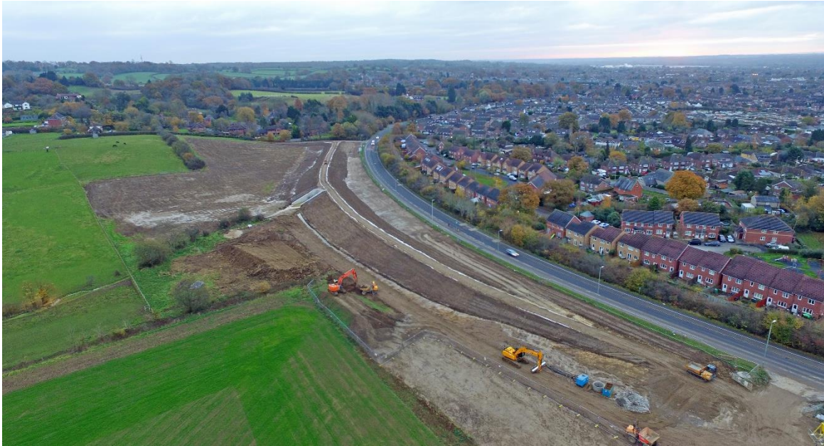
Figure 4-6: Construction phases of Tull Way Flood Alleviation Scheme (photo credit: West Berkshire Council)
