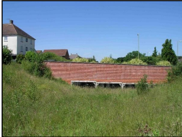
Tunnels under the roads at Marnel Park in Popley allow Great Crested Newts to move through the development
