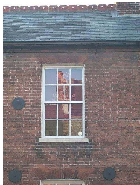
A good example of discreet upper floor advertising which is accompanied by a brass plaque at ground level
